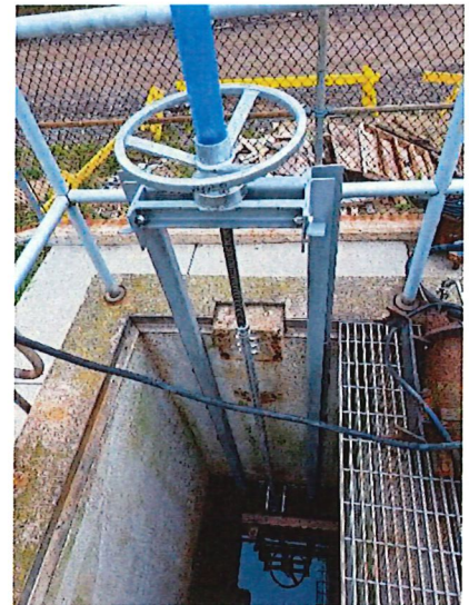
Figure 3 New Slide Gate at UV Channel
