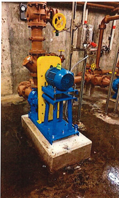
Figure 4 New RAS Pump
